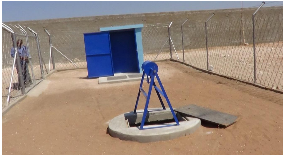
A pump station complete with its winch at Nkurenkuru
